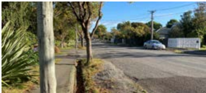
Slater St Needing Rebuild
